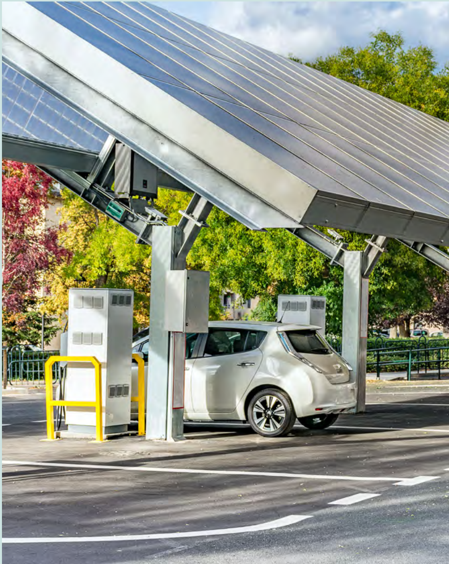
Spain: Car charging station for self-sufficient and first free photovoltaic panels in Europe.
